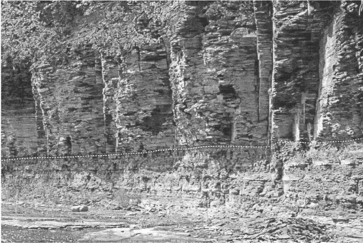
Fig. 28: Tall, close-spaced NW joints at the contact (dotted line) of the Dunkirk shale and underlying Hanover gray shale along Eighteenmile Creek.
