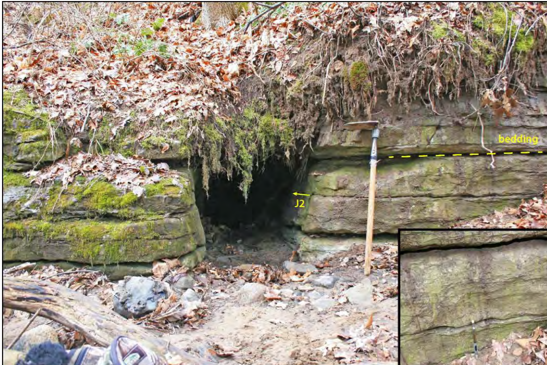
Figure 1-20. Small cave opening (28 inches (71 cm) wide by 32 inches (81 cm) high) located along the channel's right bank just upstream from culvert 2. Entrenching shovel is 32 inches long. Bedding ( 021^{\circ} 10' NW) dips away from the viewer. The cave opening follows a large solution cross-joint (J2 - 114^{\circ} ) about 5 feet (1.5 m) across a sediment-filled floor before it drops another 3 feet (1 m) into a very small passage. The Onondaga here is noncherty, thin to medium bedded, very fine-grained limestone. In places (inset photo taken to the right of shovel, mechanical pencil for scale), wavy, silty laminae parallel bedding. On weathering surfaces these stand out in greater relief compared to the more limy beds that weather out in negative relief. Photo by R. Witte.
