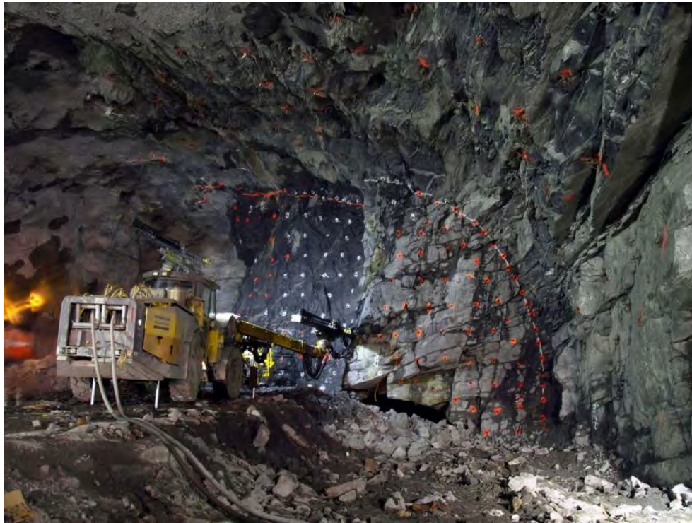
Figure 12 - View from north of west (R) and center (L) slashes of North Cavern excavation at 86 th Street Station for Second Avenue Subway. West (southbound) TBM tunnel crown at +77.2' exposed in right center of image below area of intersecting joints, faults and resulting overbreak. The center (wet, blackish area) and western (right of center) slashes are discussed in text. (Digital image taken 19 December 2012.)
