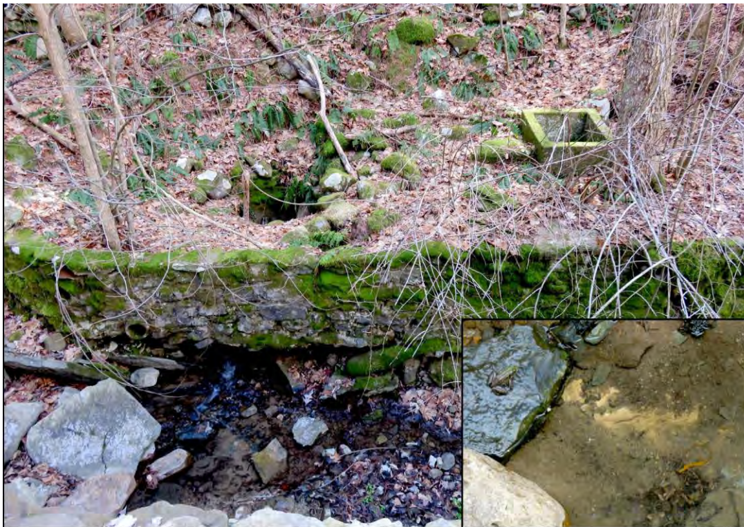
Figure 1-21. Small spring located just downstream from culvert 2. Over the years the low reservoir wall has been undercut resulting in the formation of a small sinkhole. Local denizens (inset photo) are the green-headed frog and orange long-tailed salamander, both common inhabitants of springs and seeps in karst areas. Spring photo by R. Witte and inset photo by Jon Inners.
