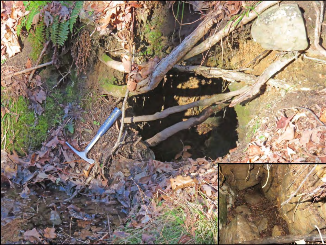
Figure 1-22. Sinkhole along right stream bank below culvert 3. Opening is 22 inches (56 cm) wide by 16 inches (41 cm) high. The subsurface cavern beneath the sink is about 4 feet (1.2 m) deep and over 7 feet (2.1 m) in length. The inset photo shows that the sink lies over a large solution channel (~ 055°). Typically, discharge from the spring upstream from culvert 3, drains into a gravelly area of alluvium near the sink. The sink has expanded over the last decade because of increased stream flow to this part of the channel, which was largely caused by the blockage of swallow holes upstream.
