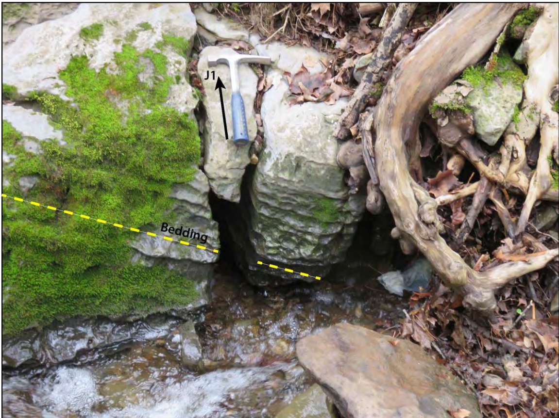
Figure 1-17. Swallow hole formed in J1 joints, located along the left stream bank and downstream from culvert 1. Water flow is from left to right, hammer for scale. Photo by R. Witte.
