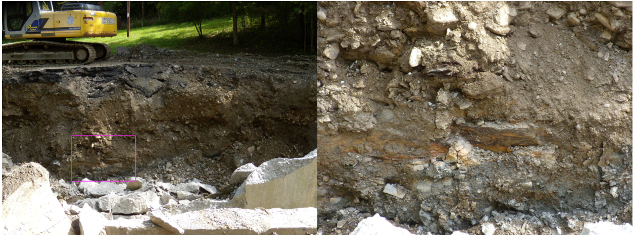
Figure 20. Subsurface beneath road a bridge under reconstruction. Area in highlighted rectangle is enlarged to the right.
