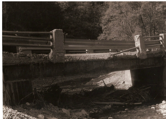
Figure 26. Old bridge, which served as a dam after debris lodged against it in 1984.
