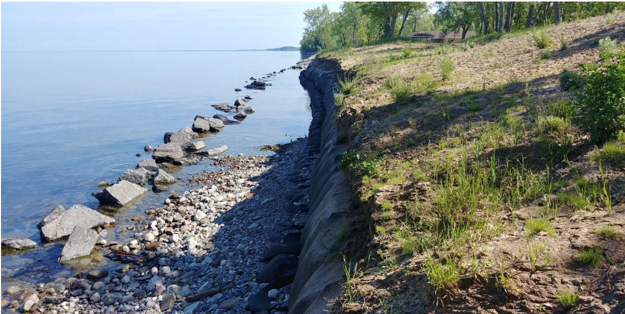
Figure 10. Failed stabilization attempt at Sandy Island Beach, 2019. Here, large, coarse rip-rap was introduced to reduce erosion of an eroding dune face, but deflected and intensified erosion-causing waves into the inadequate upland sediment (not suitable for dune material) resulting in an immediate and excessive loss of shoreline material.
