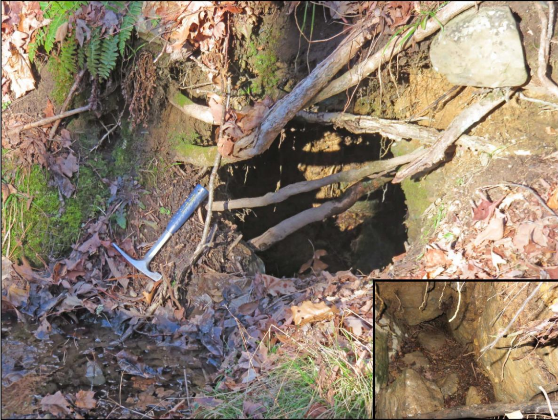
Figure 1-22. Sinkhole along right stream bank below culvert 3. Opening is 22 inches (56 cm) wide by 16 inches (41 cm) high. The subsurface cavern beneath the sink is about 4 feet (1.2 m) deep and over 7 feet (2.1 m) in length. The inset photo shows that the sink lies over a large solution channel (~ 055°). Typically, discharge from the spring upstream from culvert 3, drains into a gravelly area of alluvium near the sink. The sink has expanded over the last decade because of increased stream flow to this part of the channel, which was largely caused by the blockage of swallow holes upstream.
