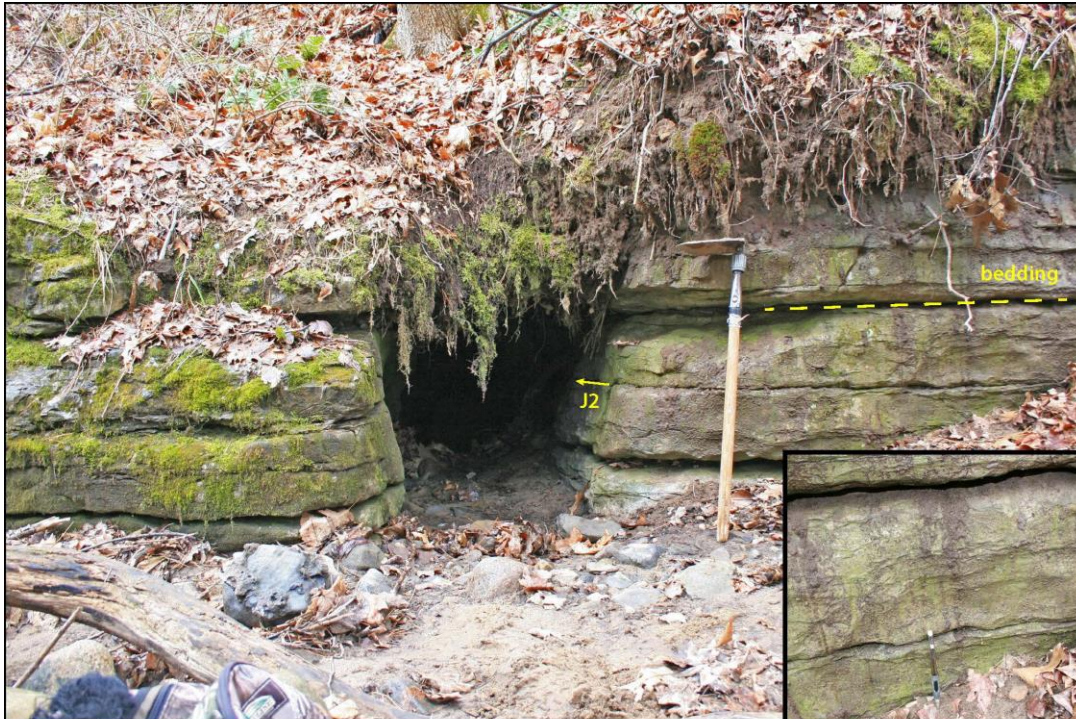
Figure 1-20. Small cave opening (28 inches (71 cm) wide by 32 inches (81 cm) high) located along the channel's right bank just upstream from culvert 2. Entrenching shovel is 32 inches long. Bedding ( 021^{\circ} 10' NW) dips away from the viewer. The cave opening follows a large solution cross-joint (J2 - 114^{\circ} ) about 5 feet (1.5 m) across a sediment-filled floor before it drops another 3 feet (1 m) into a very small passage. The Onondaga here is noncherty, thin to medium bedded, very fine-grained limestone. In places (inset photo taken to the right of shovel, mechanical pencil for scale), wavy, silty laminae parallel bedding. On weathering surfaces these stand out in greater relief compared to the more limy beds that weather out in negative relief. Photo by R. Witte.
